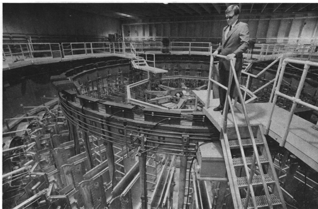
DURING SATURN CONSTRUCTION, Jim Powell (1230) surveys progress in converting PBFA I into the new X-ray-producing accelerator.
